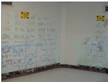
As a result of a steam leak, these walls offer a glimpse of the past.
